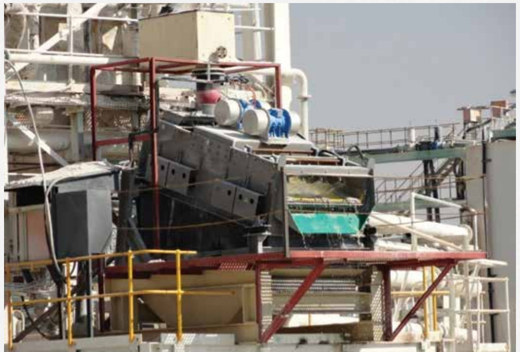
Figure 2: A Virto-Cuccolini RS2814.1 installed at a silica mine in South Africa
